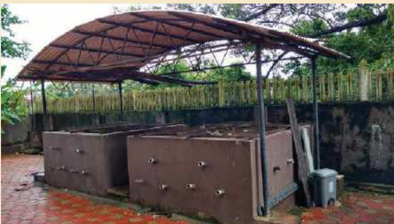
Photo 7.8c Decentralized Composting Units in Panaji, India
