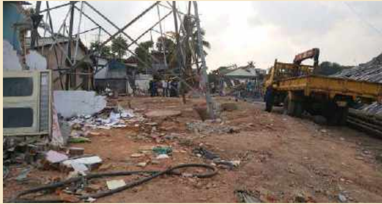
Photo 7.6 Recovery Efforts after Meethotamulla Dumpsite Collapse from Heavy Rains in Colombo, Sri Lanka
